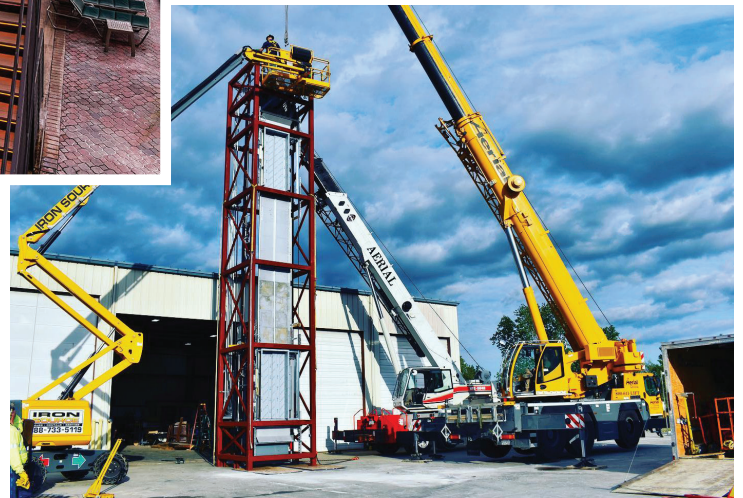
UPS AND DOWNS: DEI's clients include The Don CeSar hotel in St. Pete Beach, Florida (above), and the National Air and Space Museum in Washington, D.C. (top). Most projects use equipment produced by the company's Delaware Elevator Manufacturing division (right).
